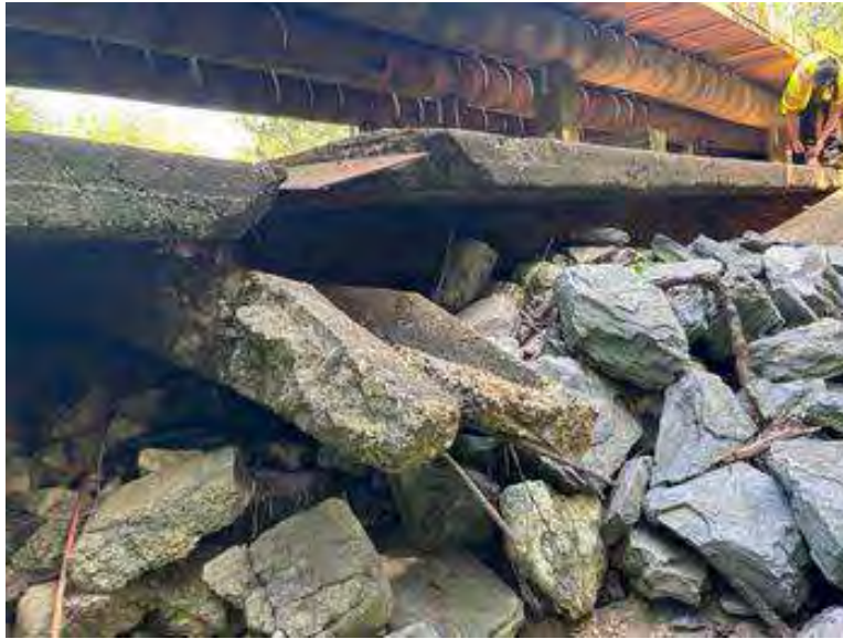
Stone fill beneath collapsed concrete spillway
