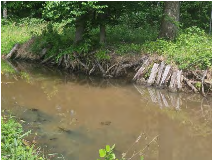
Erosion along Northern Bank
