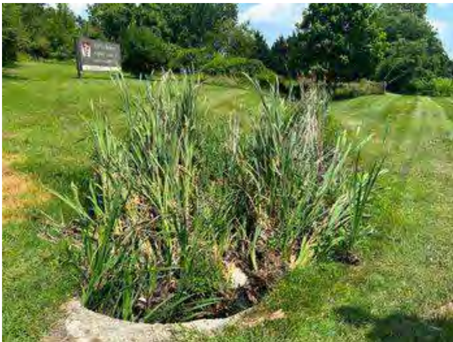
Overgrown Vegetation Blocking Inflow
