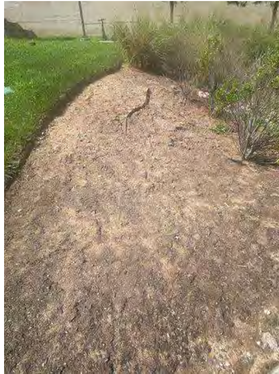
Bare area on slope
