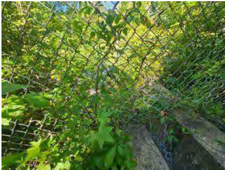
Tree growth on embankment.
