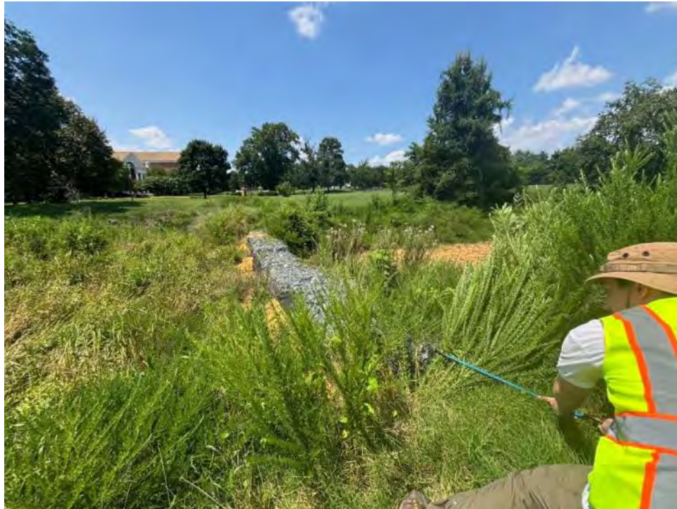
Gabion basket between west forebay and treatment basin
