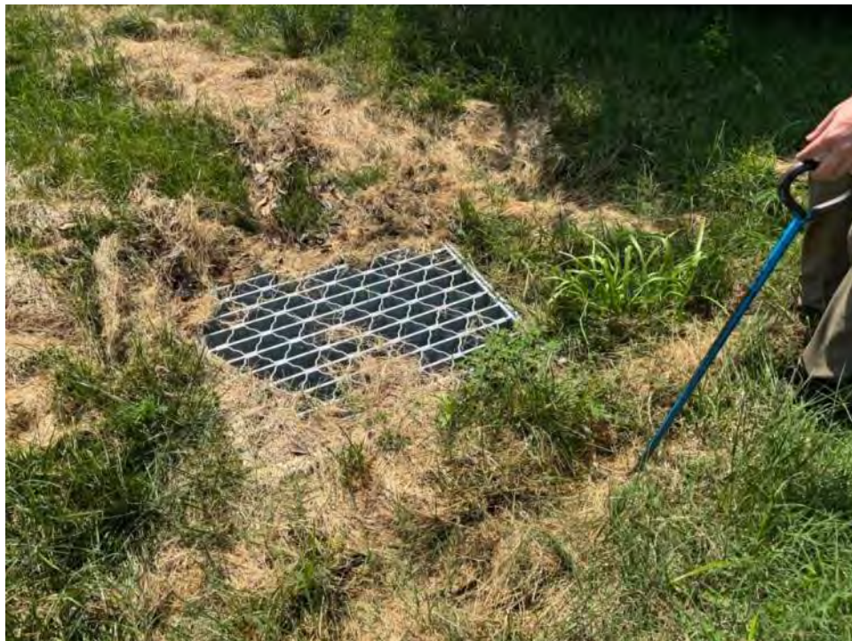
Small hole forming around control structure
