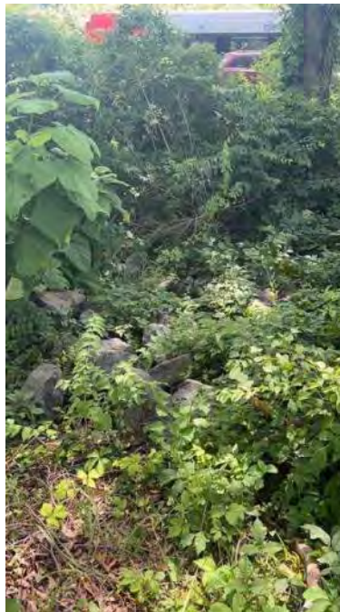
Overgrown Rip Rap 1
