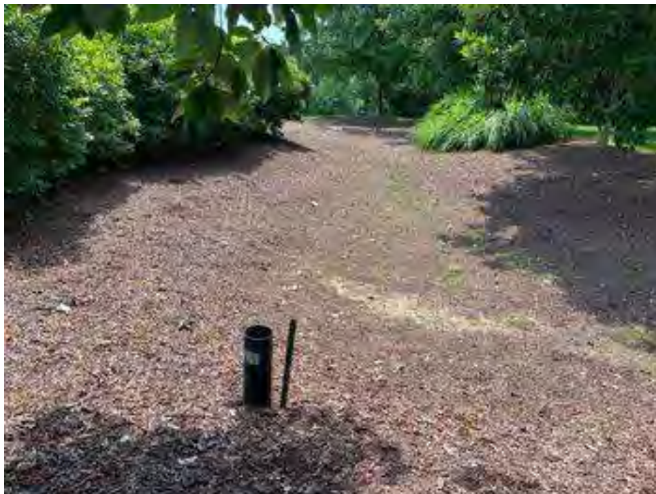
Minor sediment erosion at upper treatment basin
