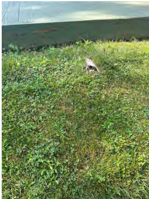
Broken inflow 1 pipe
