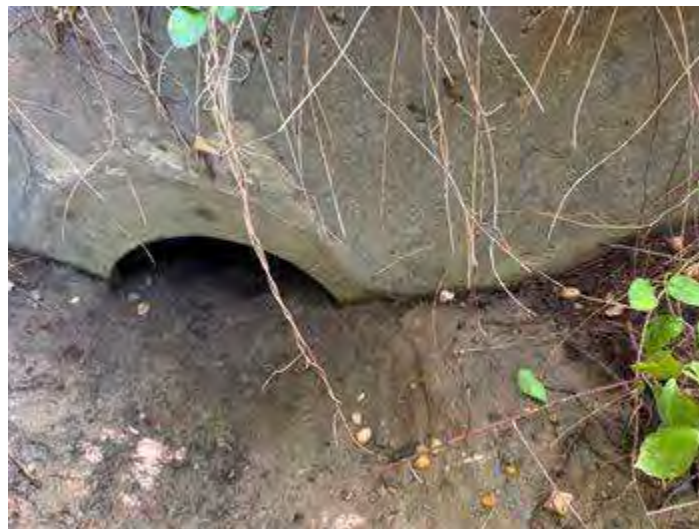
Clogged outflowing pipe
