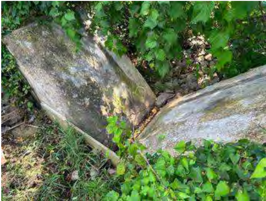
Control Structure with Low Flow Orifice Blockage
