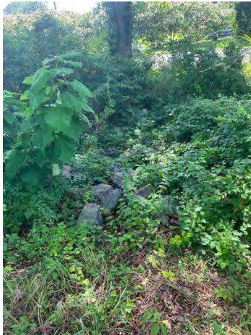
Overgrown Rip Rap
