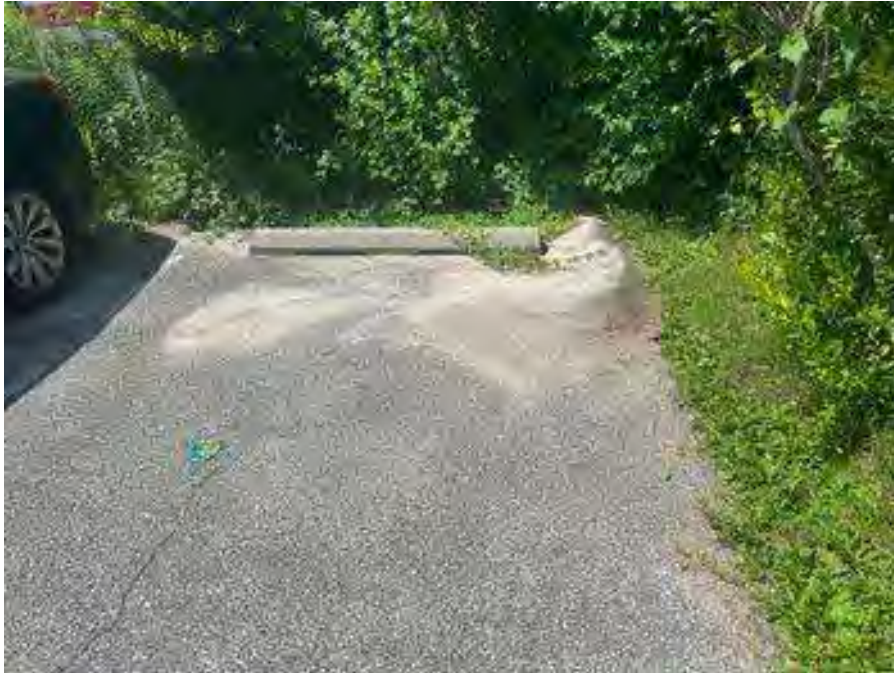
Minor Sediment Buildup in Sheet Inflow 2
