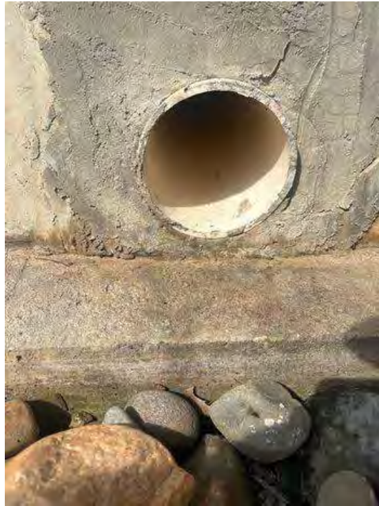
Pipe at inflow
