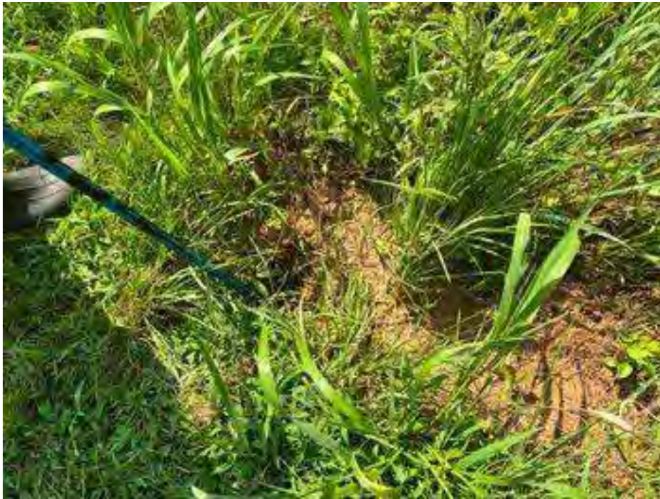
Small eroded channel on berm
