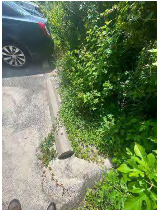
Minor Sediment Buildup in Sheet Inflow 1
