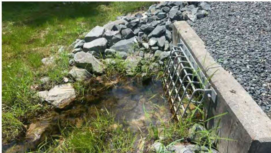
Trash Rack with Ponding
