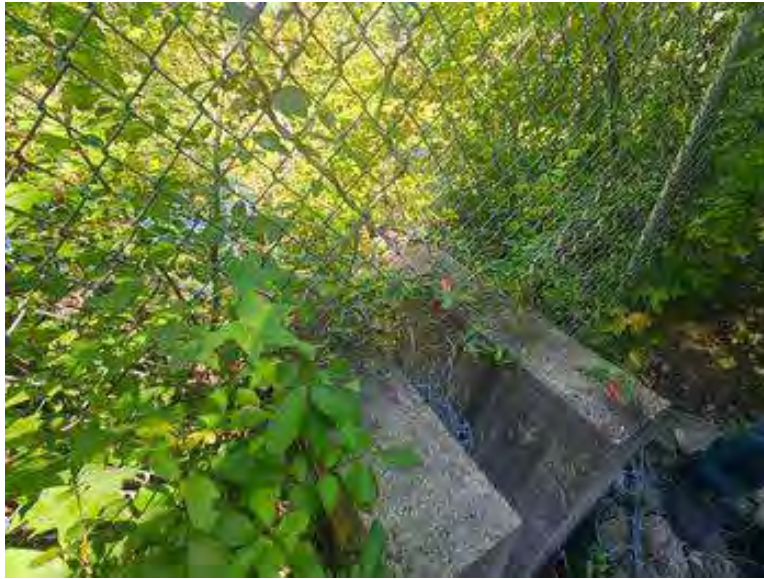
Tree growth on embankment.
