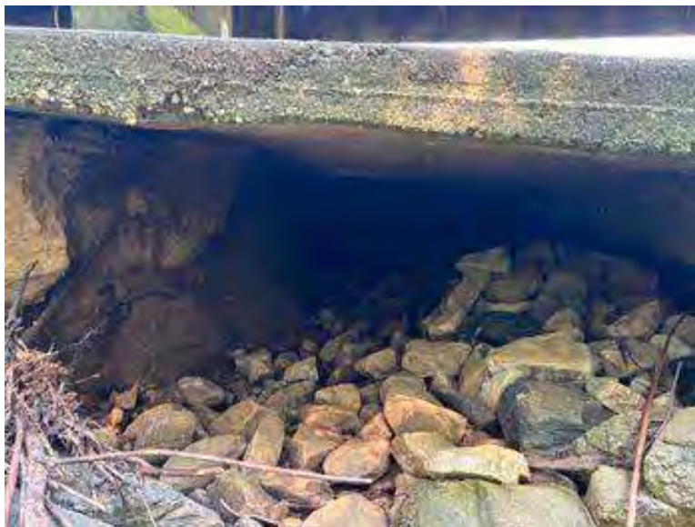
Stone fill beneath collapsed concrete spillway
