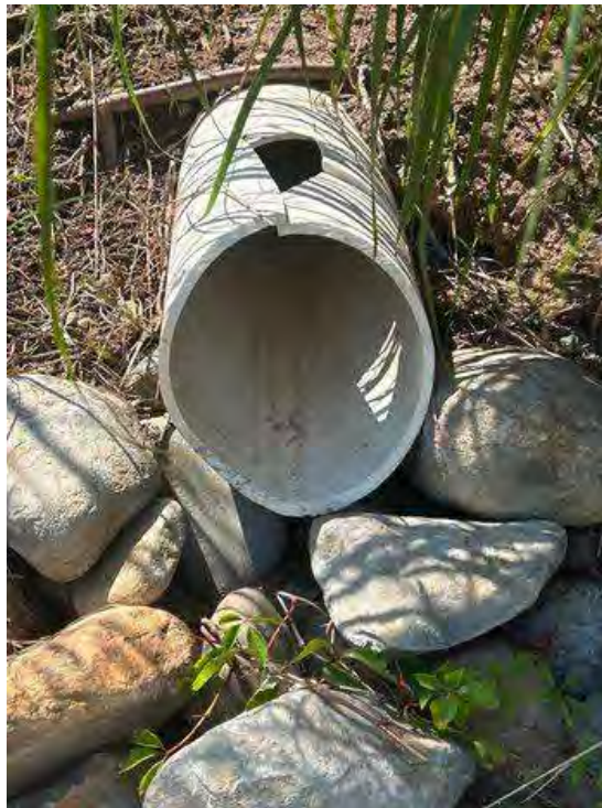
Damaged inflow pipe
