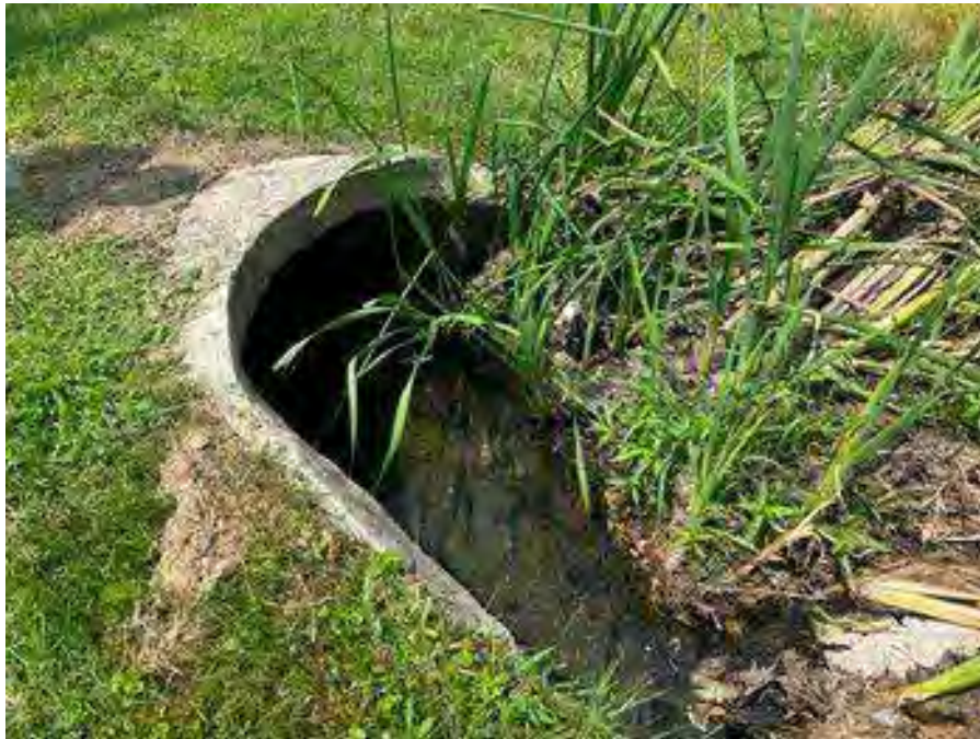
Inflow Close Up with Overgrown Vegetation
