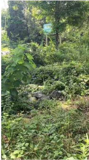
Overgrown Rip Rap 2
