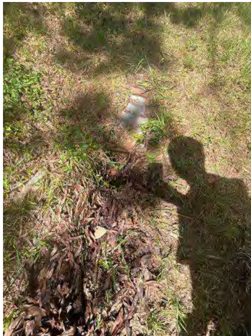
Collapsed Inflow Pipe Close Up
