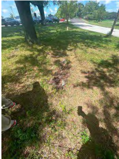
Collapsed Inflow Pipe Overall
