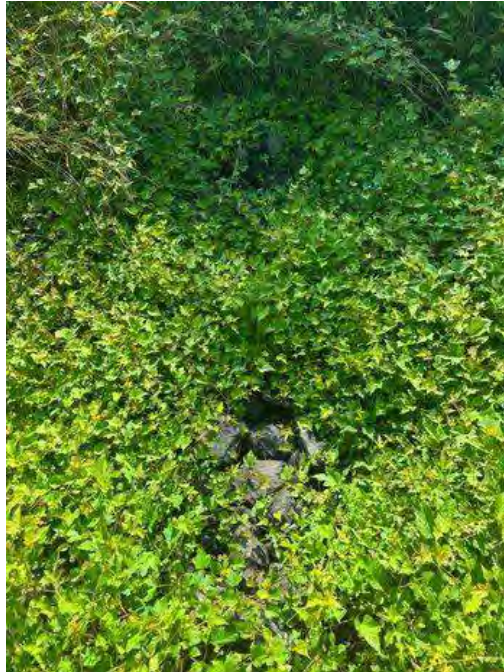
Overgrown Rip Rap Close Up
