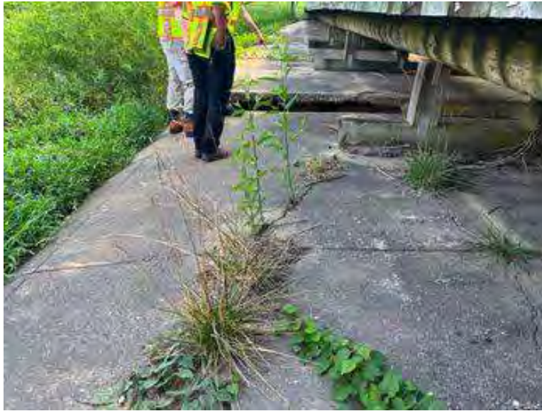
Cracks within concrete spillway. Golfcart path constructed on top.
