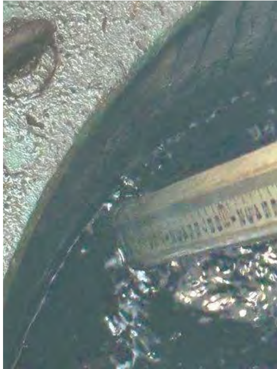
Water surface within stormceptor
