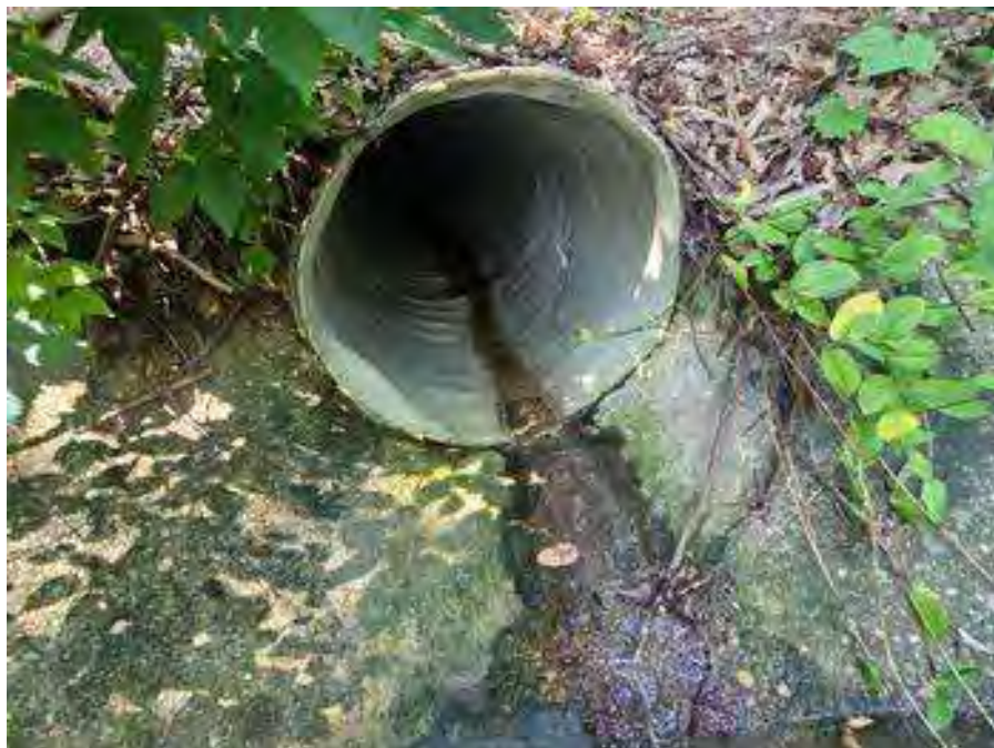
Inflow 1 with Active dry weather flow Close Up
