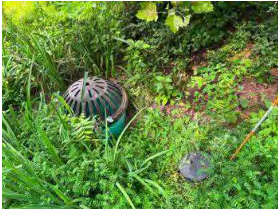
Control structure and monitoring well
