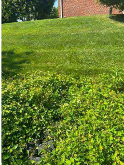
Overgrown Rip Rap
