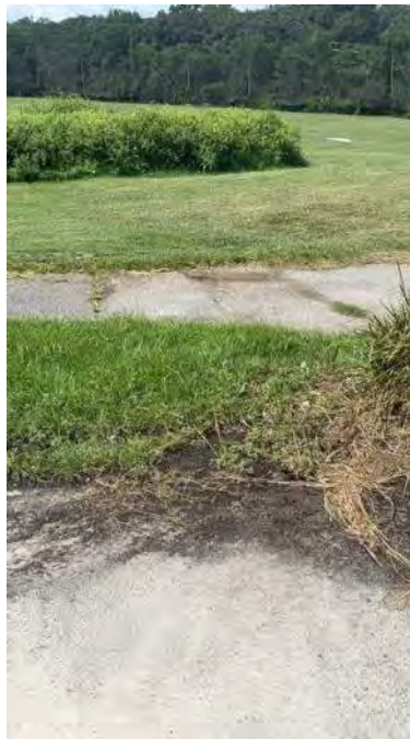
Sediment Buildup Near Rain Garden
