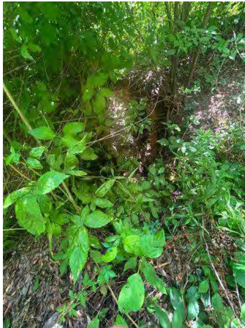
Eroded Channel Near Outfall 2
