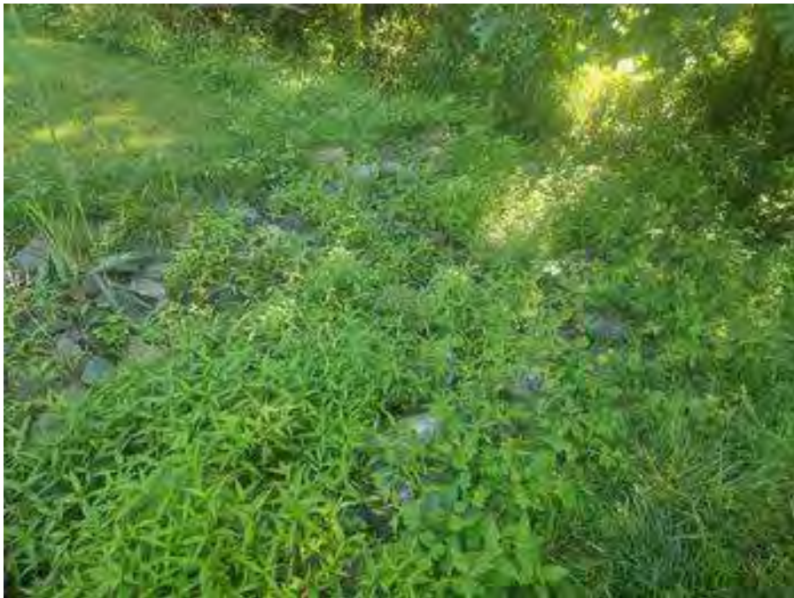
Overgrown Vegetation in Rip Rap
