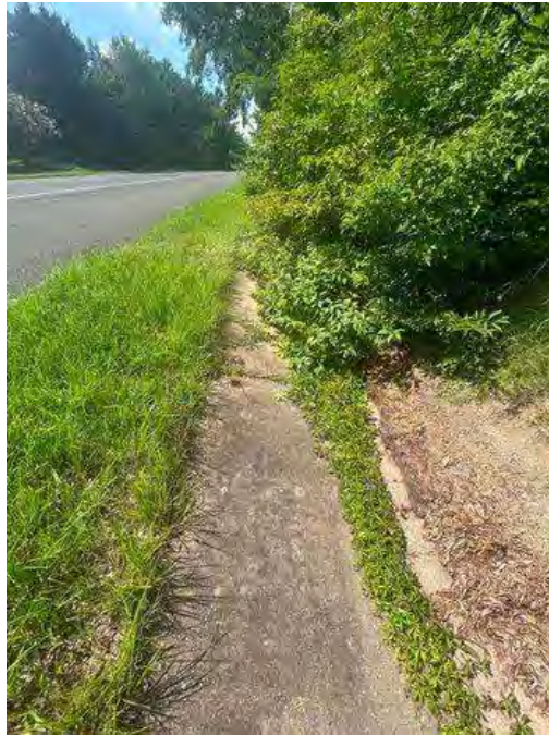
Cracked Outfall Entrance
