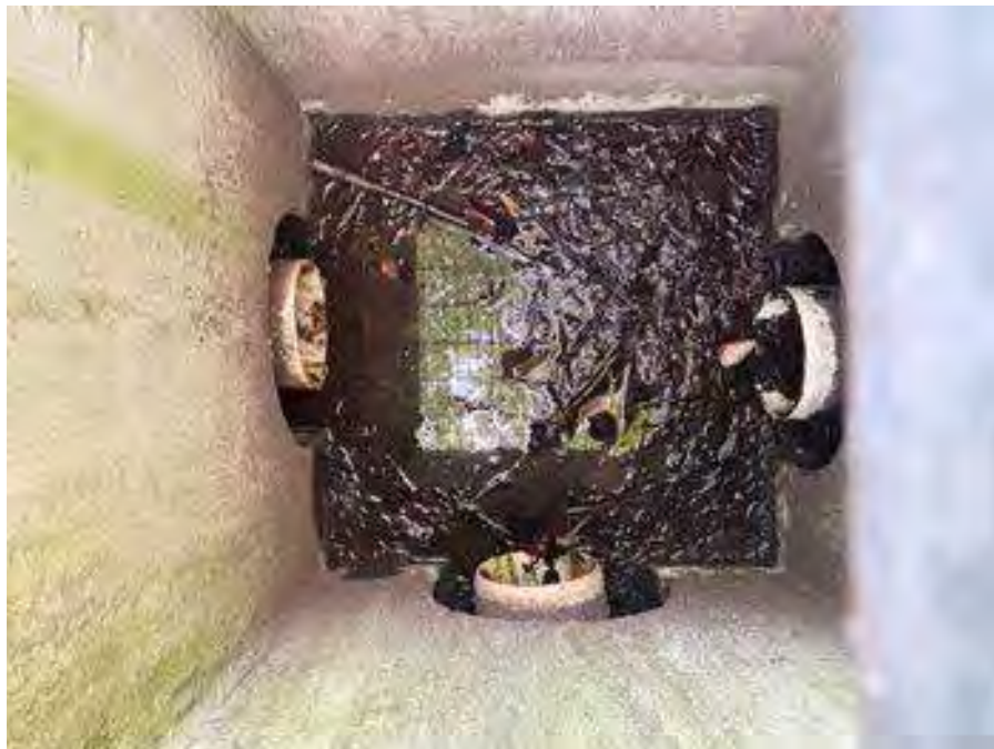
Control Structure Interior with Debris Buildup
