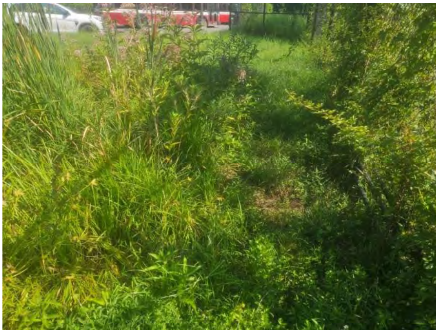
Principal Spillway with Erosion
