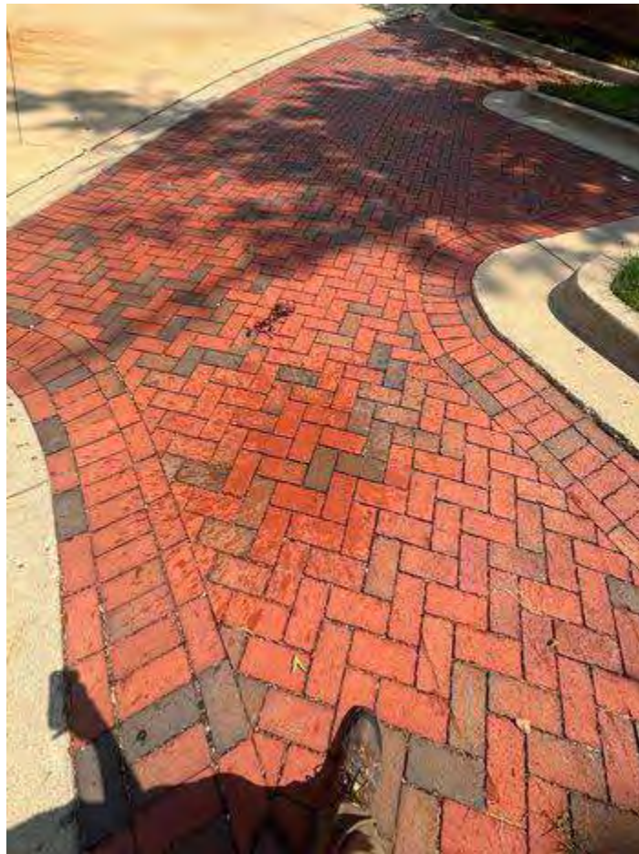
Water permeating into surface
