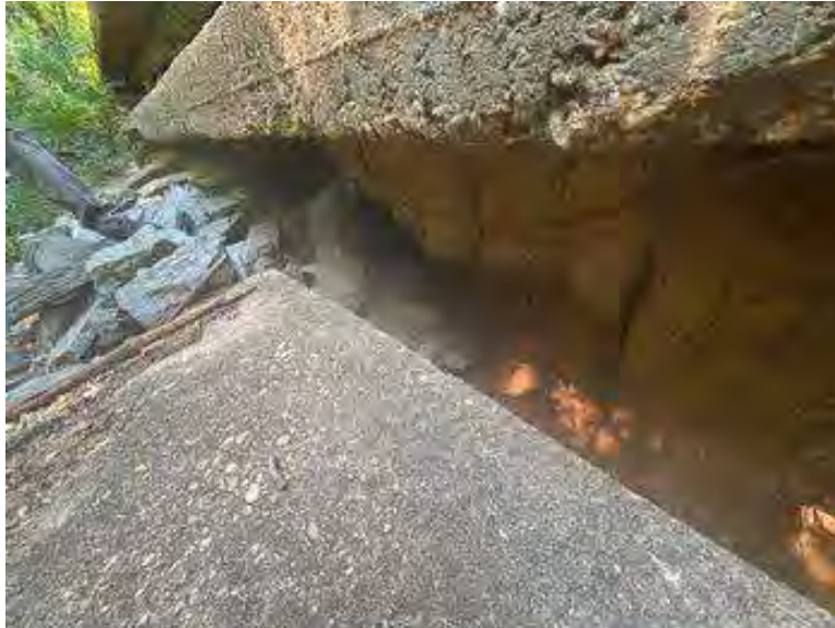
Collapsed concrete spillway
