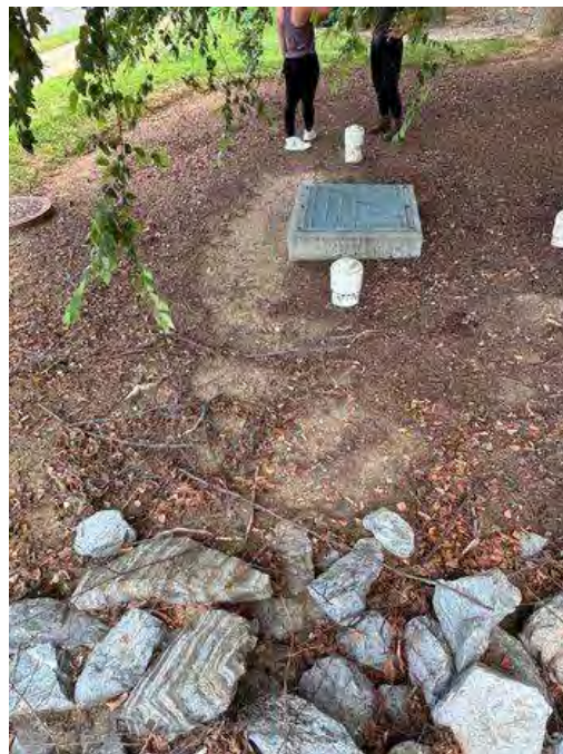
Control Structure Overall and Minor Erosion
