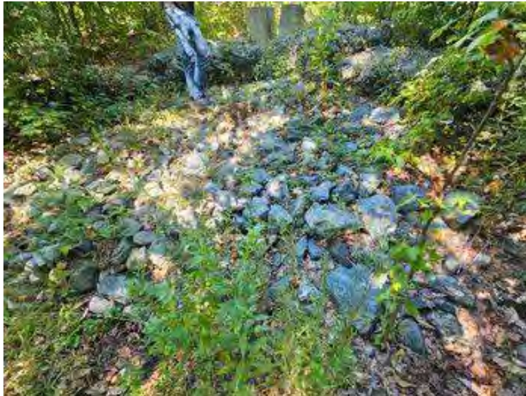
Outfall. Minor vegetation and debris.
