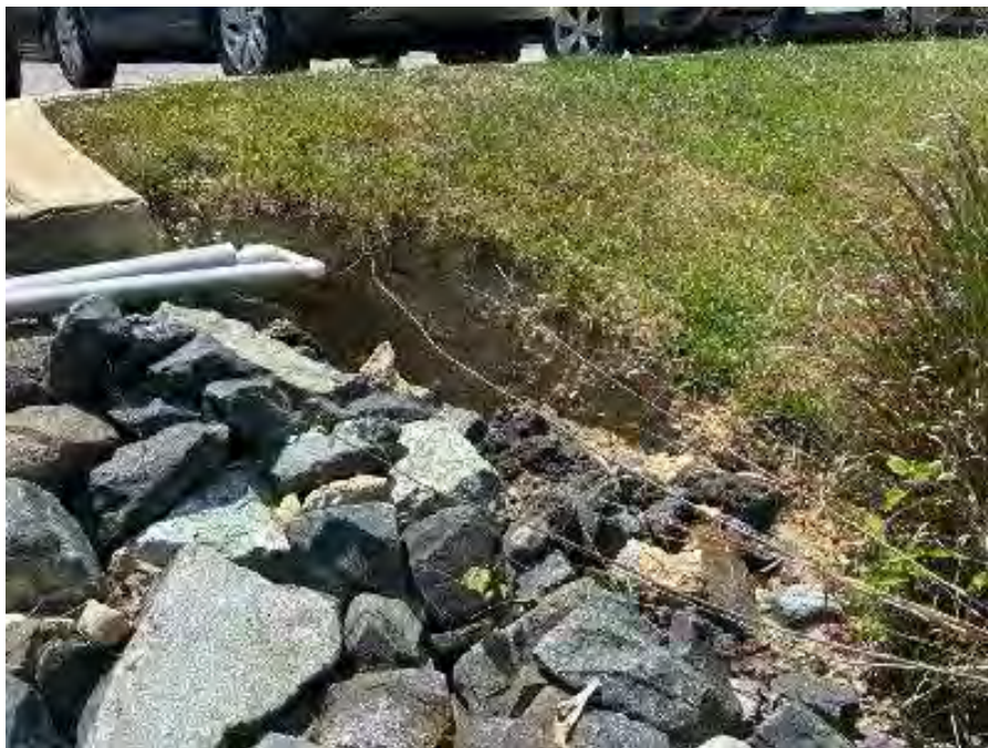
Erosion Occurring to Inflow
