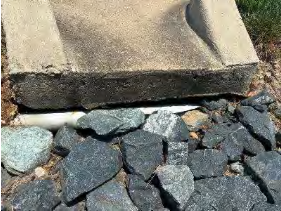
Exposed Pipe at Inflow
