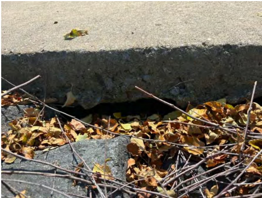
Erosion Occurring to Inflow
