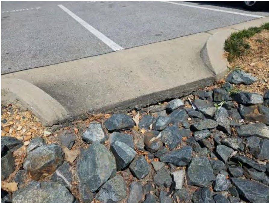
Erosion Occurring to Inflow
