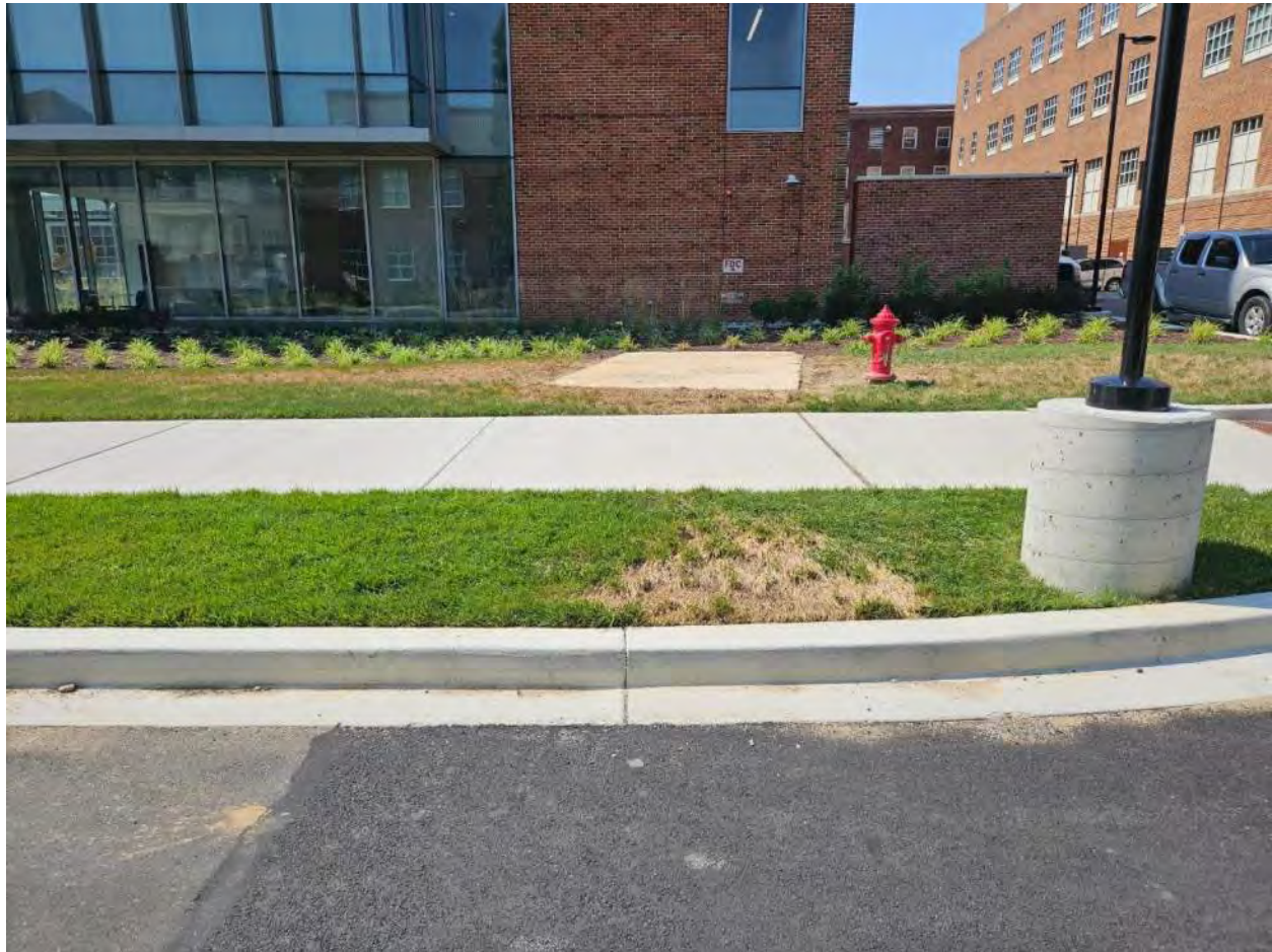
Erosion Affecting Grassy Area
