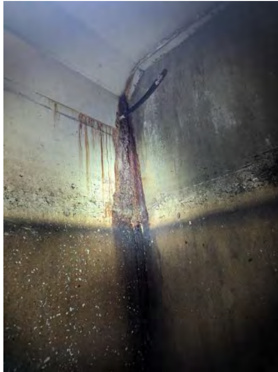
Discoloration on structure wall
