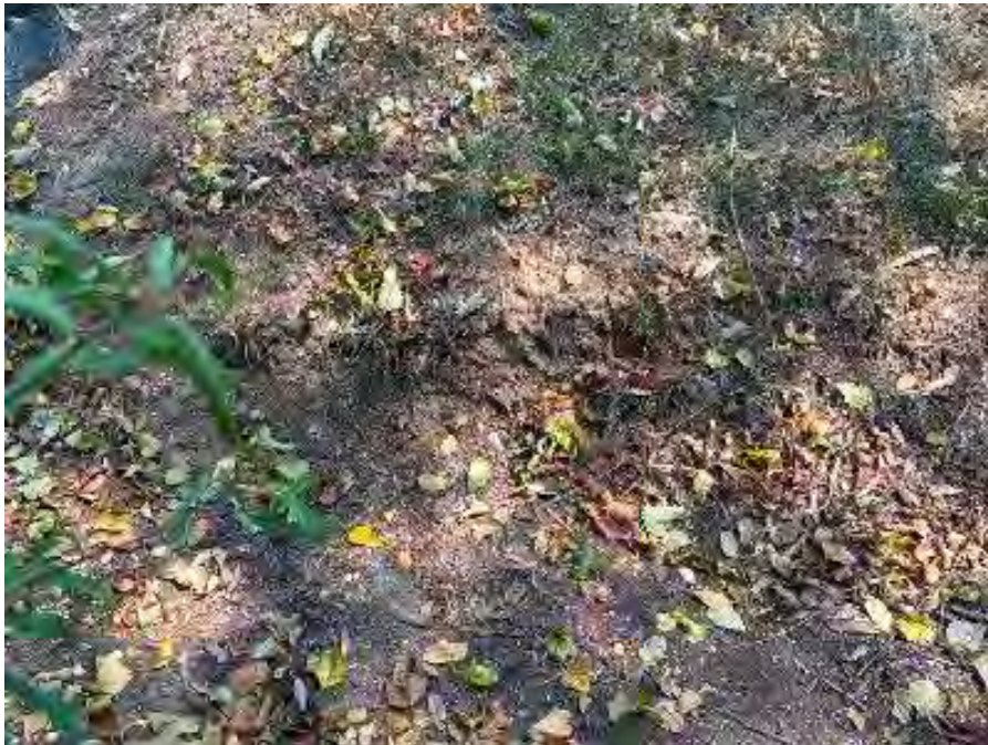
Slight Erosion Occurring to Embankment
