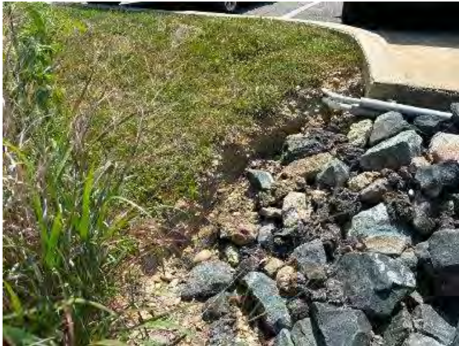
Erosion Occurring to Inflow
