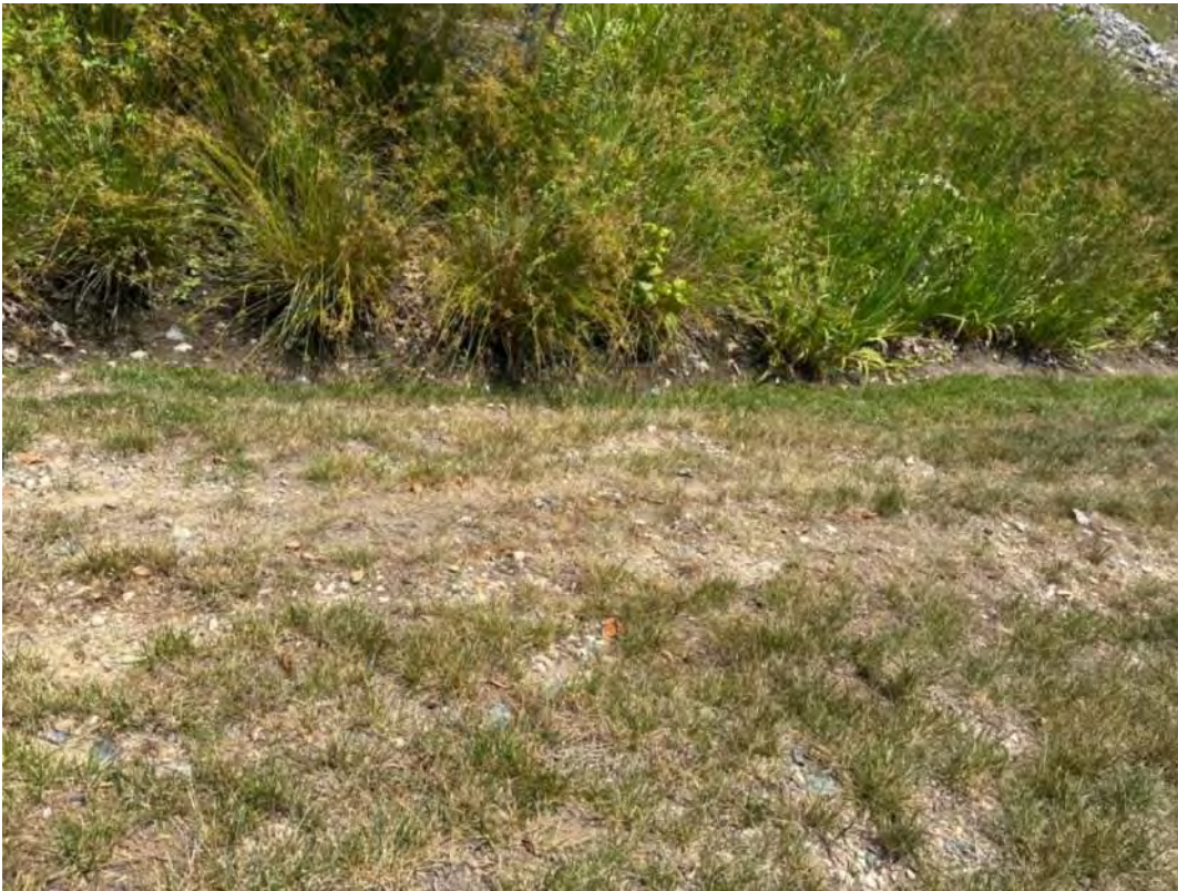
Erosion Occurring to Embankment
