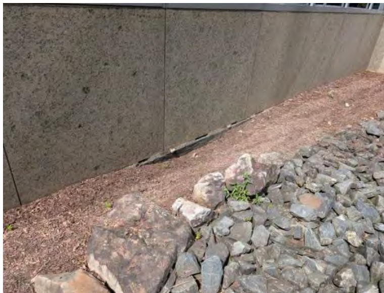
Erosion at building
