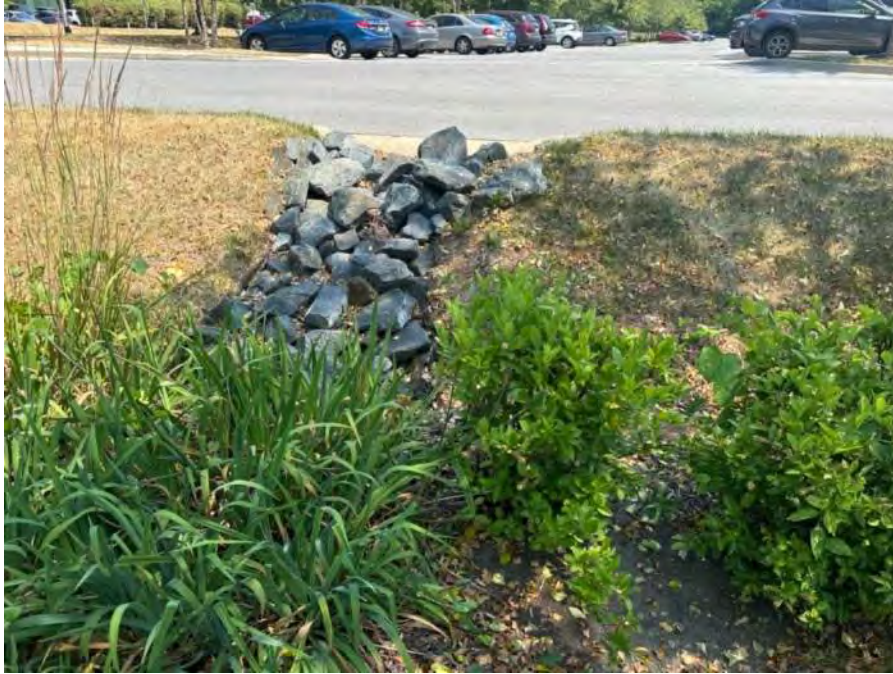
Vegetation Obstructing Inflow
