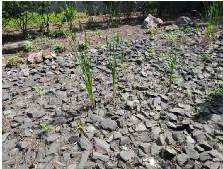
Vegetation growth in riprap
