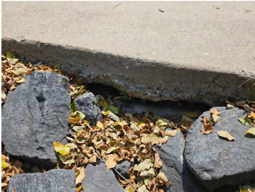
Erosion Occurring to Inflow
