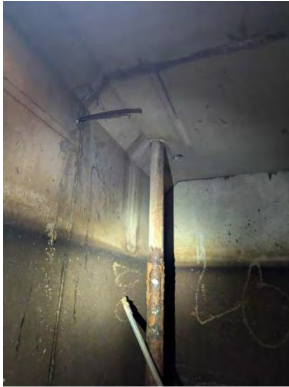
Connection pipe to irrigation
