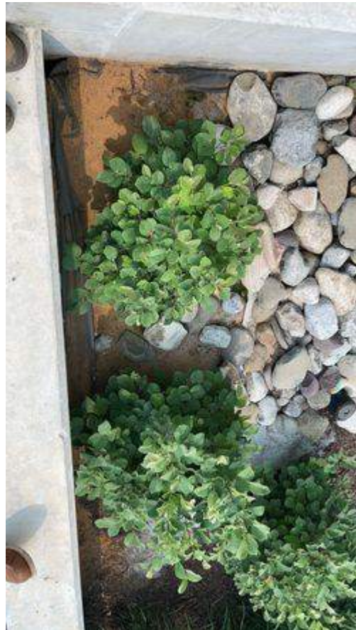
Sedimentation at inflow:
