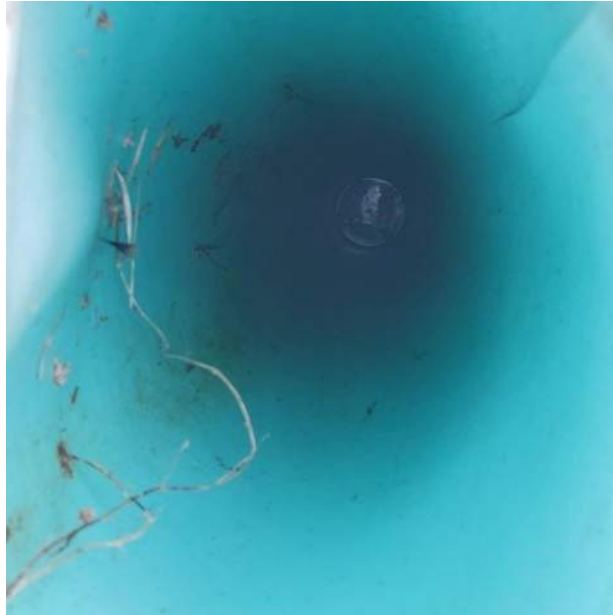
Cleanout 1 – Standing water
