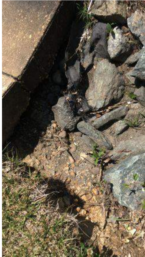
Erosion around culvert. Potential damage
